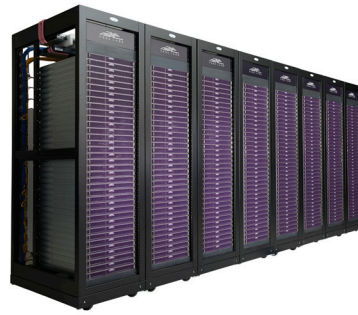
FIGURE 2 | Data Center Rack
